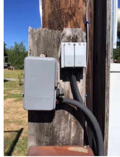
Timer box (locked) and light switches
